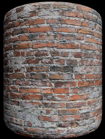
Bricks & Sloppy Mortar 12
