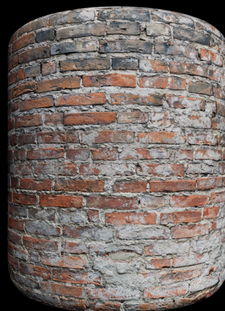
Bricks & Sloppy Mortar 22
